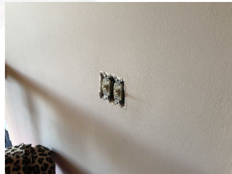
Missing cover, 2nd floor
