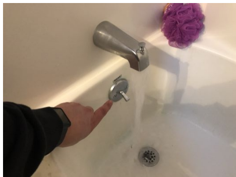
Stopper was not working on 1st floor bath tub
