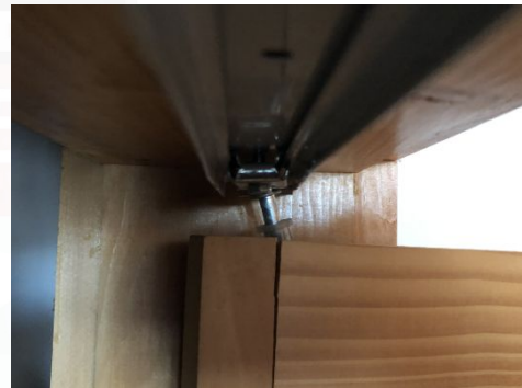
2nd floor closet door's hardware appeared damaged.
