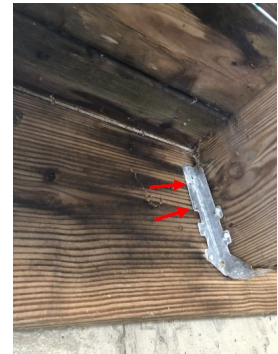
Missing nails in joist hangers
