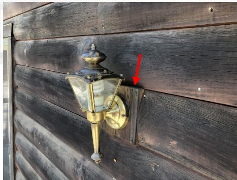
Head flashing should have been installed
