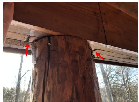
Irregular framing of porch header observed
