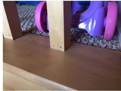
It appeared that the balusters were installed with brad nails, this is not the normal why to install them.
