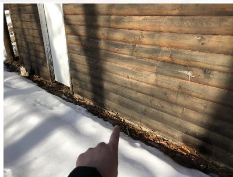
Log siding was below ground level, wood rot was observed
