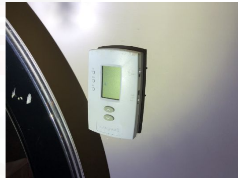
Unit in basement had a dead battery. This caused the zone in the basement to not able to turn on and was not inspected.
