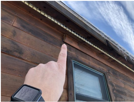
Loose log siding
