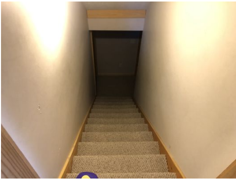
Missing railings on basement stairway
