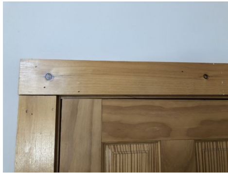
Note: Door to basement rubbed on frame
