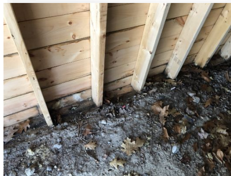
Wall system under porch area had major wood rot, untreated lumber was used.
