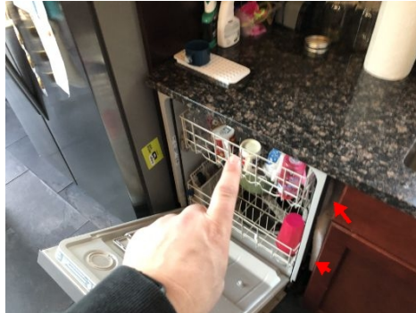
Dishwasher had not be installed or secured properly.
