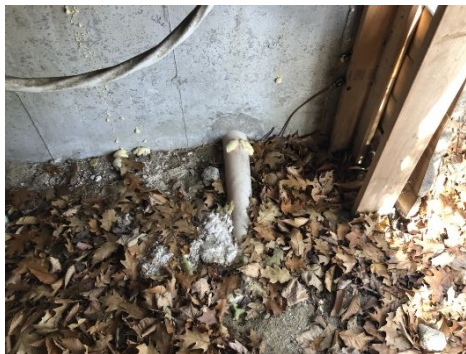
Recommend covering with gravel to insulate and protect
