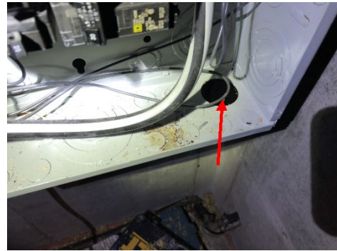
Knock out was missing and needs to be closed off.
