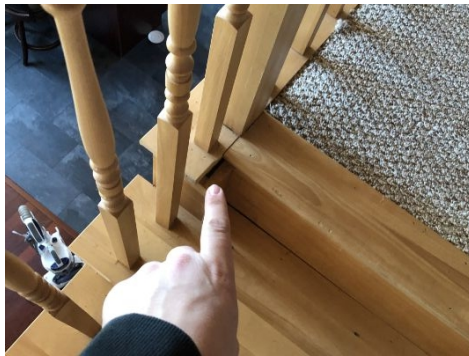
Cracked/missing trim on stairway
