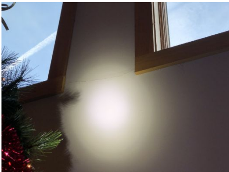
Small crack observed, common
