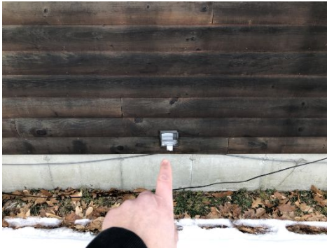
Dryer vent appears to be taped shut
