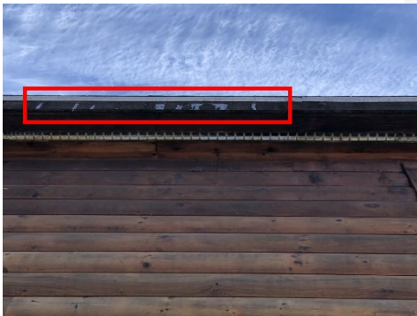
Some deterioration observed on fascia board
