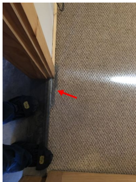
Carpet was lifting in 1st floor bedroom
