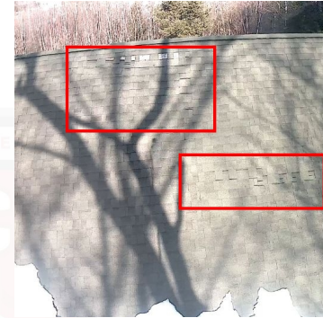
Numerous shingles missing and loose. Likely an active leak.
