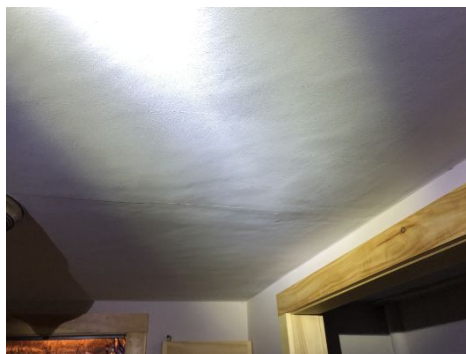
Small cracks and staining observed in basement ceiling.
