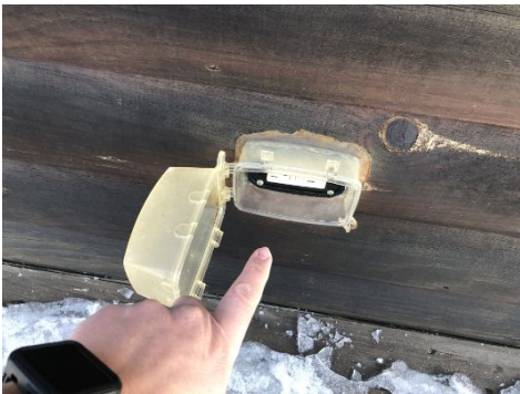
Both outside outlets did not appear to have power and the outlet would not reset. Recommend replacement/repair
