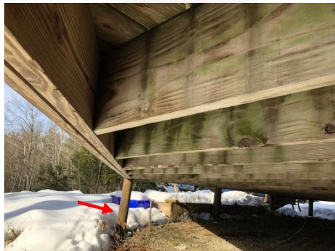
Recommend updating to proper support posts. 6" by 6" pressure treated post with footing was recommended.
