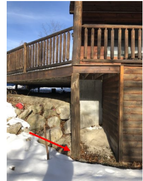
Wood rot observed
