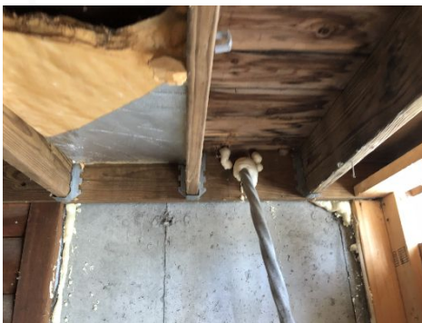
Missing lag bolts on ledger of porch
