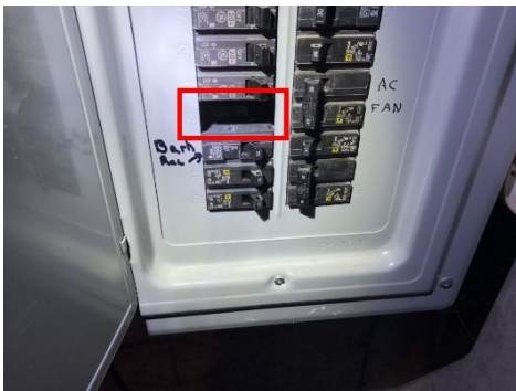
This opening needs to be closed off. Safety hazard.
