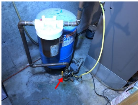
Shut off location
