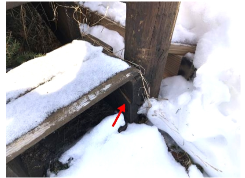
Broken stair stringer, this is causing the railing to be unstable
