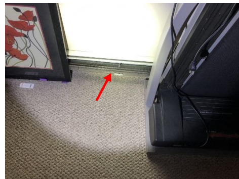
Missing baseboard cover
