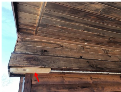
Past repair observed to soffit, may have been to block a pest entry point
