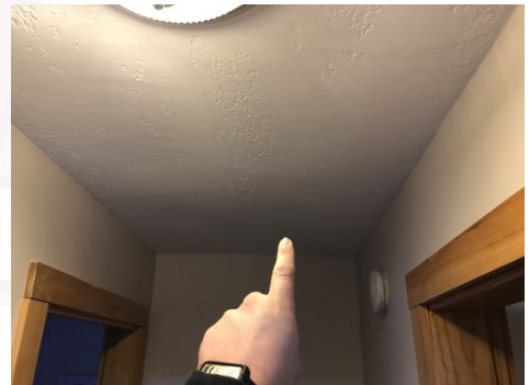
Small sag in ceiling observed, unknown reason
