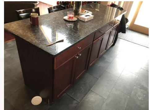
Missing GFCI outlet on island, this is recommended for today's standards
