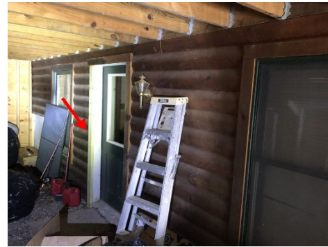
Past wood repair observed
